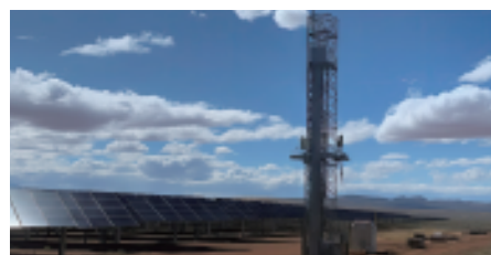
Telecom Tower Solar System
